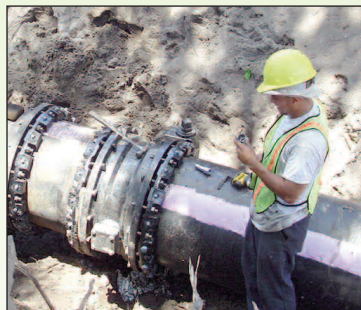
With its water reclamation project, Delray is helping to conserve fresh water from the area's aquifers.
